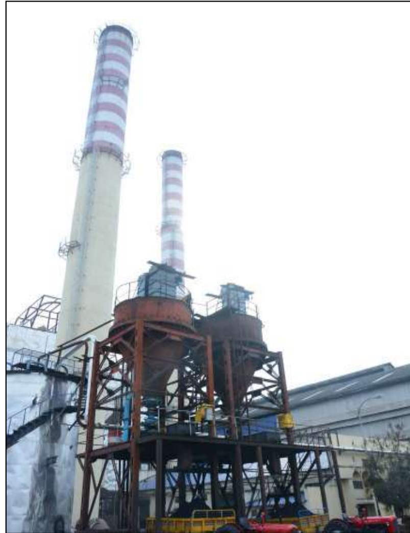
Boiler Ash Handling System
